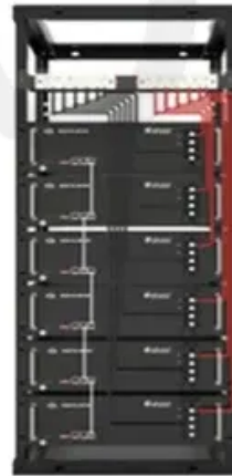
Cabinet and rack installation display
